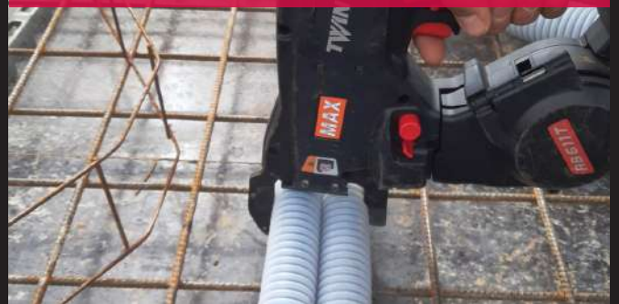
Electrical and plumbing piping
